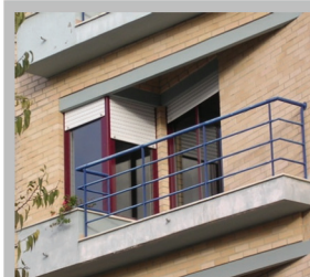
Dangerous distance between bars
